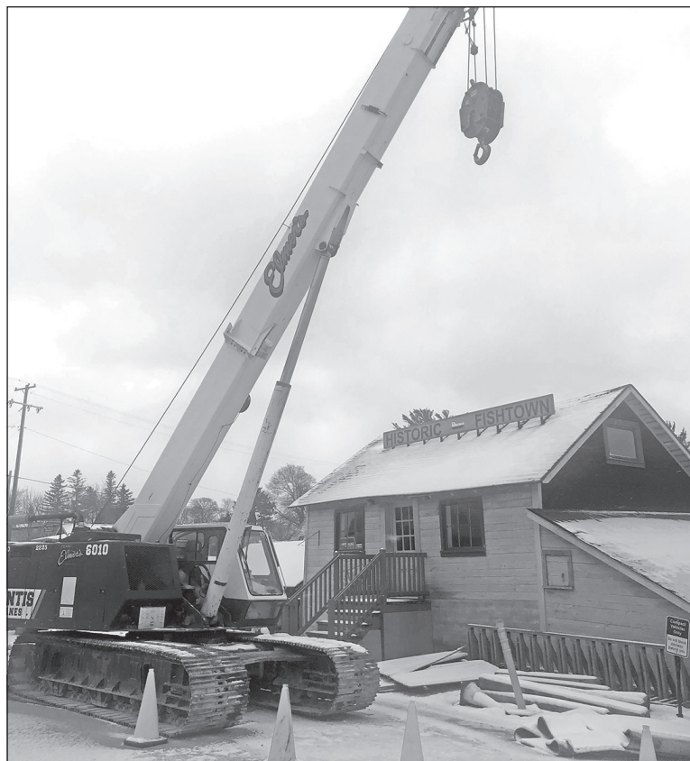
Inclement weather slowed work earlier this week in Fishtown, with cranes owned by Elmers put on standby. Biggs Construction is the general contractor. Enterprise photo by Alan Campbell
